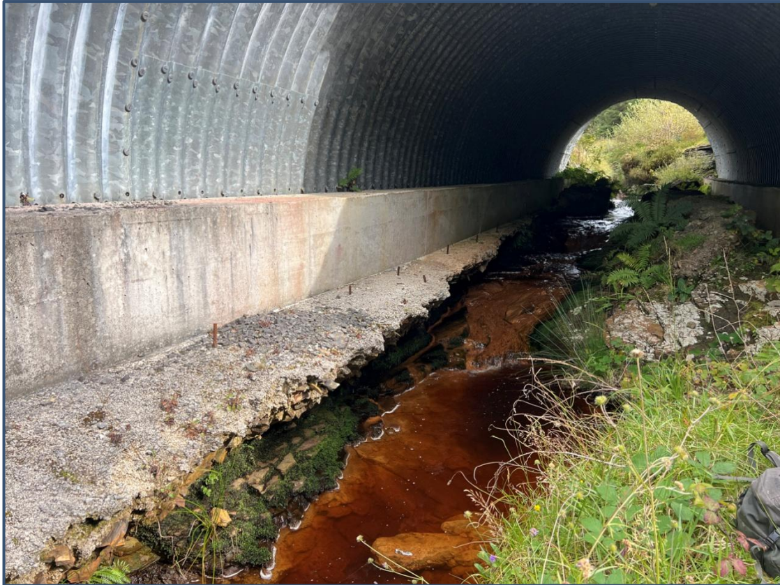
Plate 4-12. Upstream-facing perspective of the watercourse as it traverses beneath the bridge which bisected the surveyed area.
