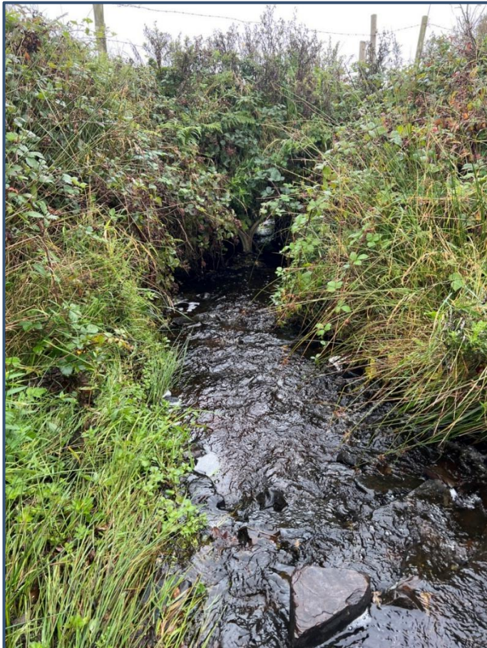
Plate 4-6. Double underroad culvert situated at the downstream extent of the surveyed area.
